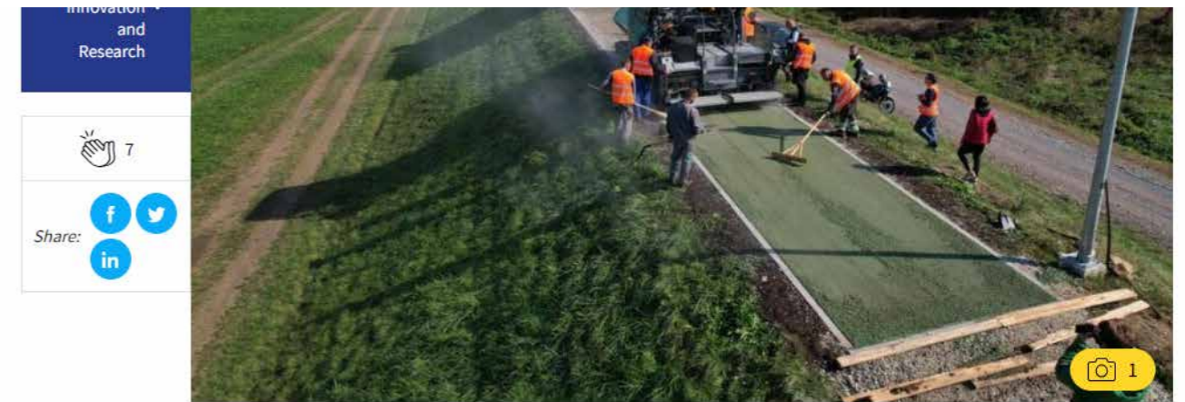
Laying down the eco-asphalt section of the Croatian Greenway, Source: City of Zagreb
